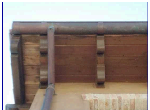
Water stains rear right
