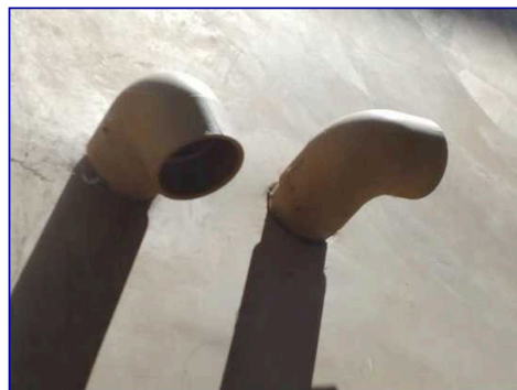
Exterior pipe voids
