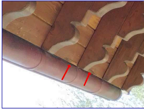
Water stains right rear
