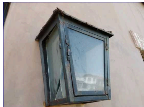
Deterioration upper right
