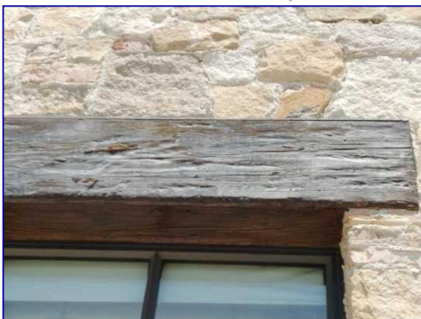
Weathered, peeling front
