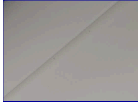
Stains right ceiling
