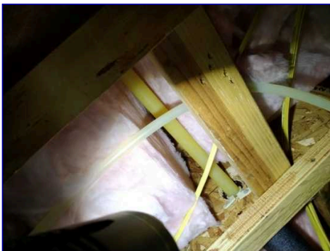
Missing insulation lower attic
