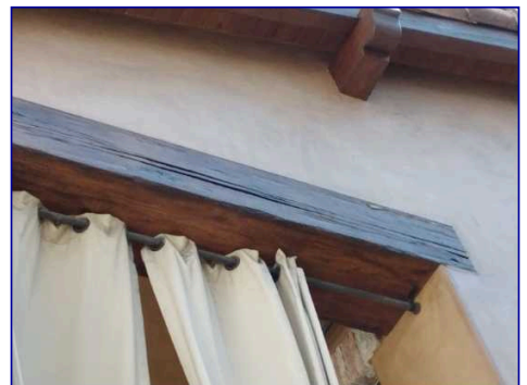
Left rear cracks, voids
