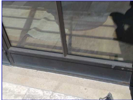
Front left rusting, weathering
