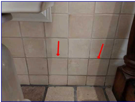
Right wall cracks
