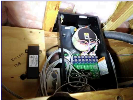
Box cover missing
