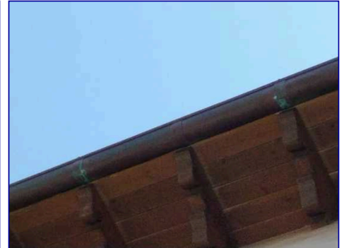
Seams leak left
