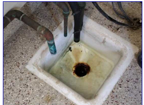
Corroded, rusting right closet
