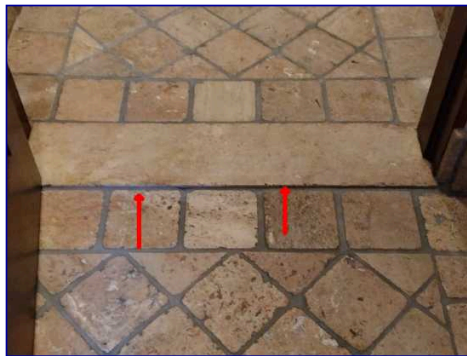
Uneven entry floor
