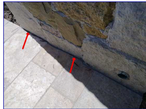
Joint cracks right
