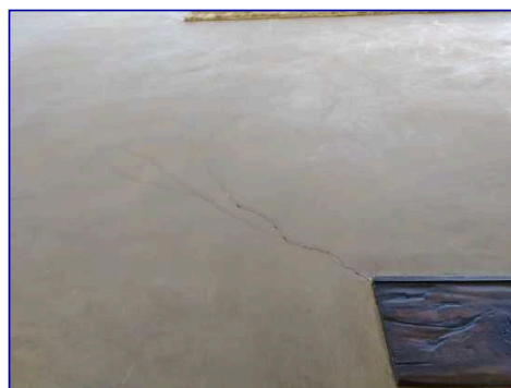
Cracks left rear
