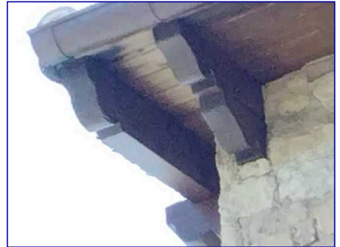
Water stains right
