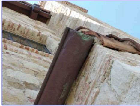
Leaking seam right
