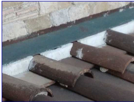
Right cement cracks
