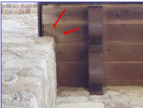
Water stains left
