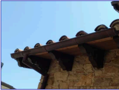
Rusting, uneven right
