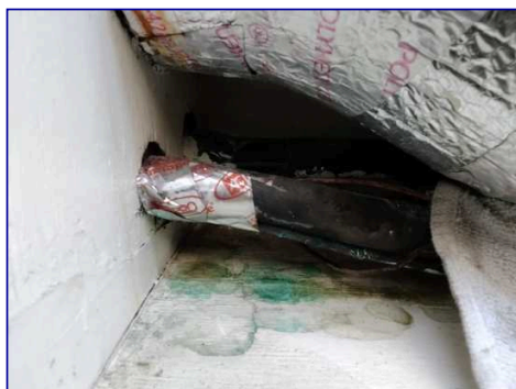
Exterior closet damage, stains
