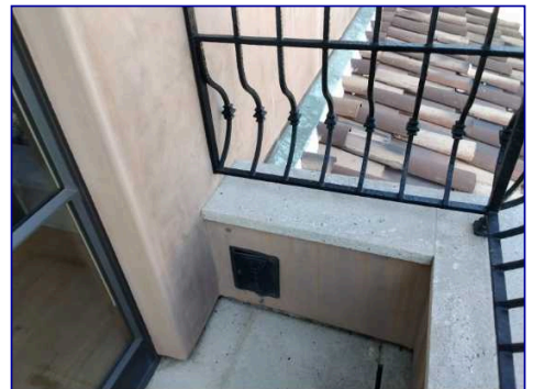
Upper right discoloration
