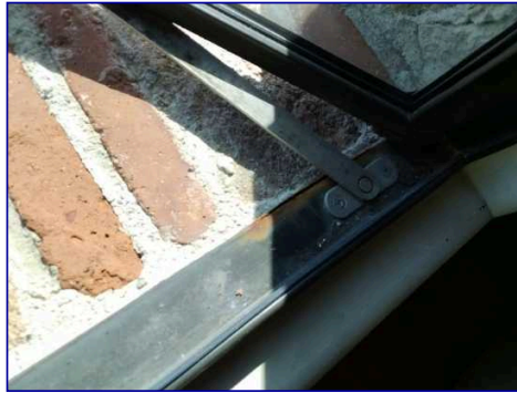
Front den rusting
