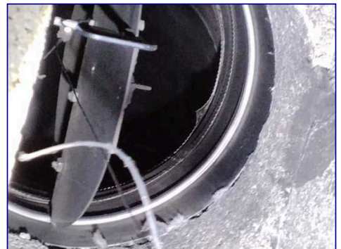
Flue bent, voids
