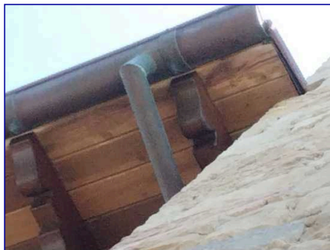
Water stains left
