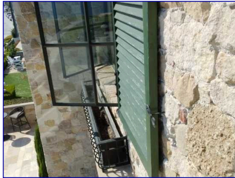
Shutters weathered, peeling
