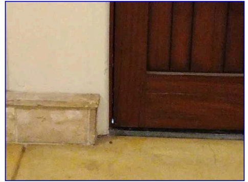
Rear poor weather stripping
