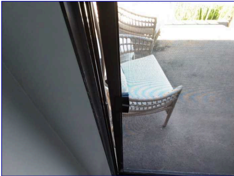
Balcony screen bent
