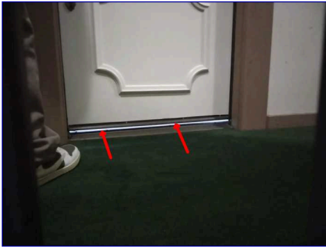
Main entry poor weather stripping
