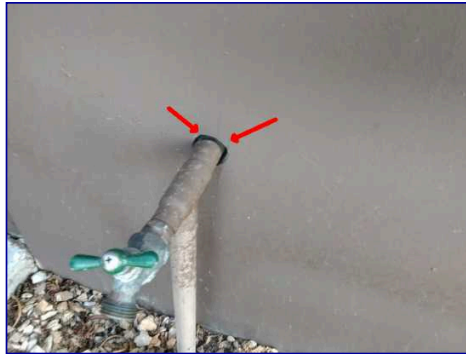
Poor caulking front pipe
