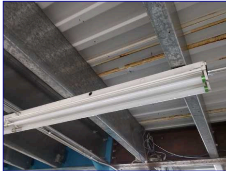
Damage light under racks
