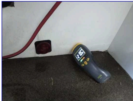
Moisture under sink
