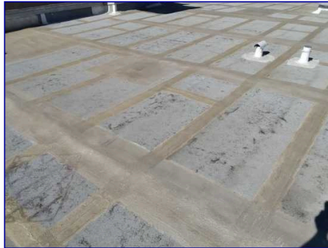
Deterioration of granules
