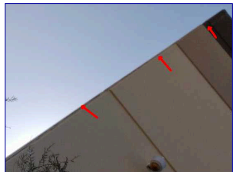
Rear left joint voids
