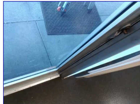
Main entry uneven
