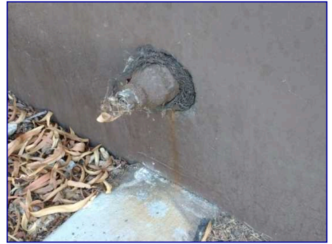
Left rear rusting, weathered
