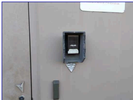
Left box cover missing
