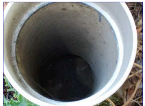
Debris, no cap
