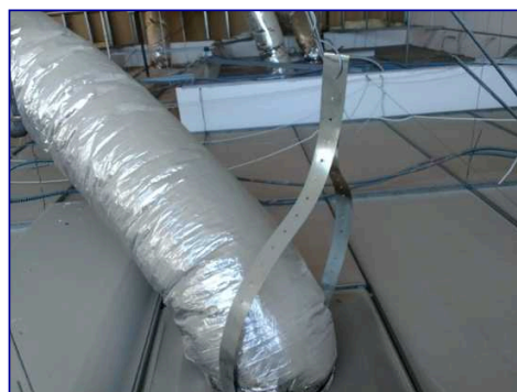
Lobby register ties loose
