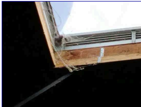
Stains near skylight
