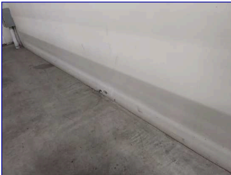
Discoloration, deterioration lower wall
