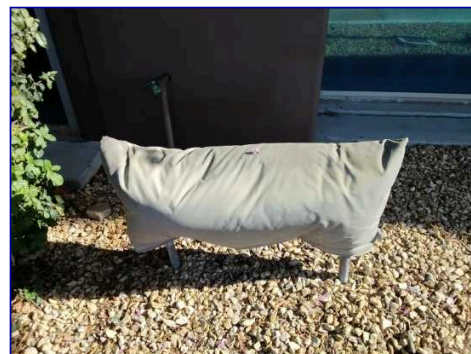
Backflow, shut off
