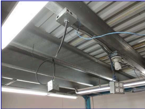
Open knock outs, damage wires
