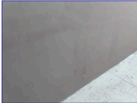
Discoloration, peeling left
