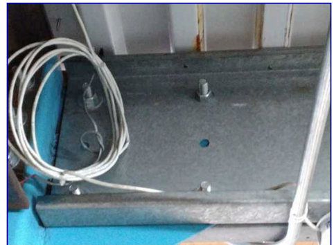
Missing washers mezzanine
