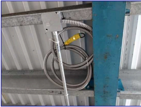
Open wire ends
