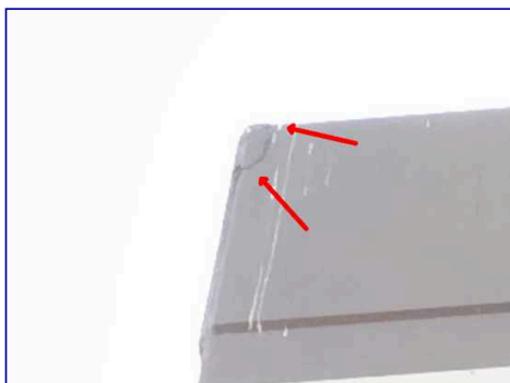
Ledt rear spalling
