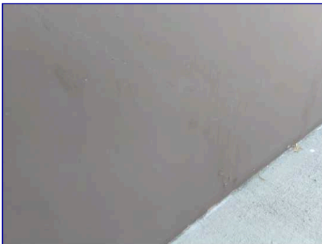
Cracks, peeling, discolored left
