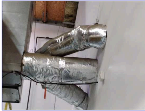
Flex ducts voids
