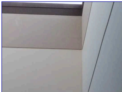
Cracks upper left
