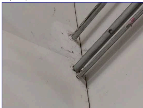
Pipe voids firewall
