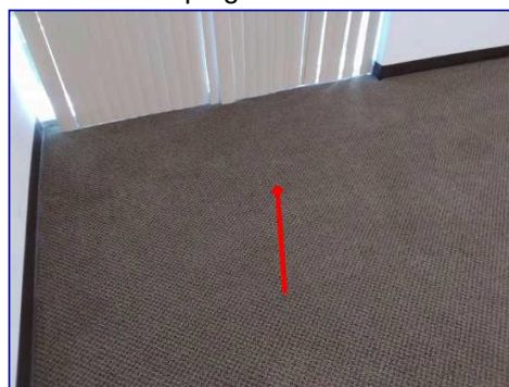
Floor uneven front office
