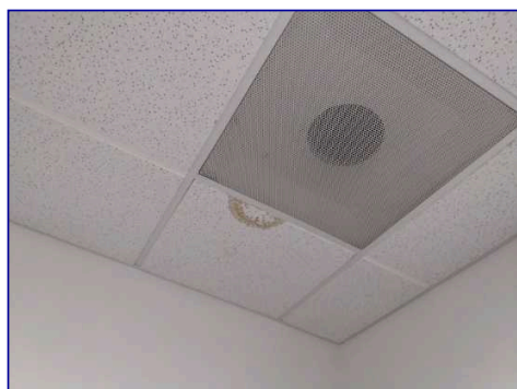
Stains rear right ceiling
