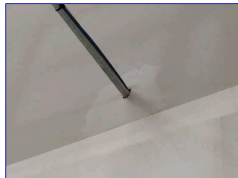
Pipe voids firewall
