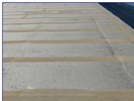
Deterioration of granules
