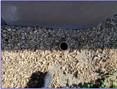
Front cap missing
