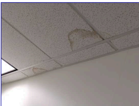
Stains hall ceiling
