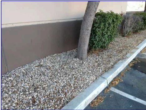
Large tree at foundation
