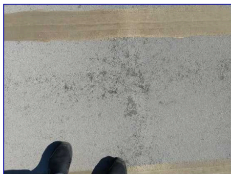
Deterioration of granules
