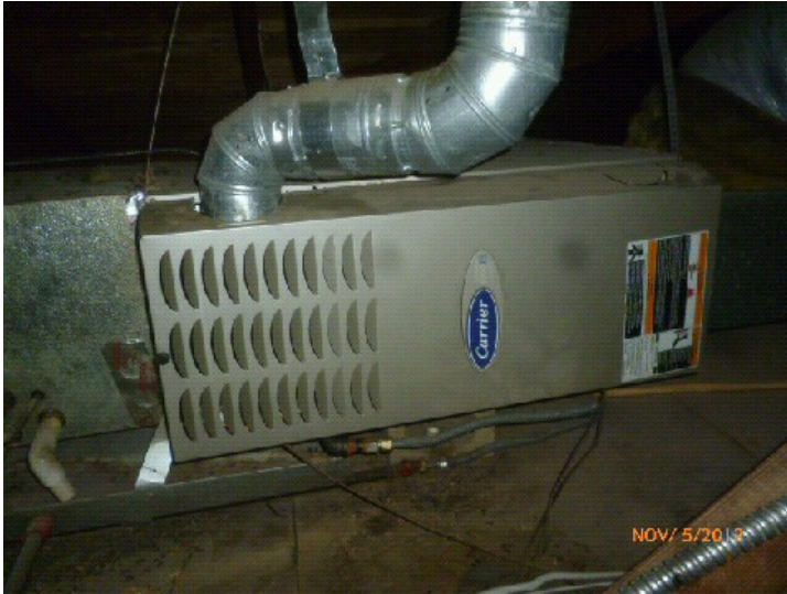
FAU in attic
