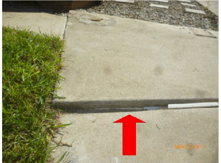
Trip hazard at front concrete walkway
