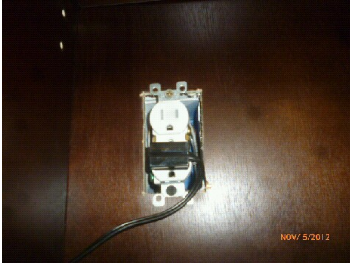
Front bedroom missing outlet cover
