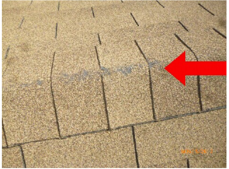
deterioration noted on roof
